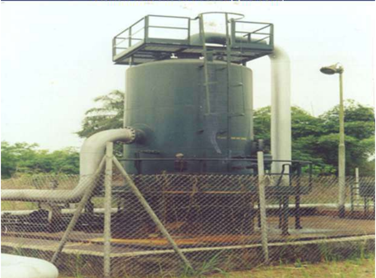
Plate 8: Flare Knockout Vessel (gas vent)
